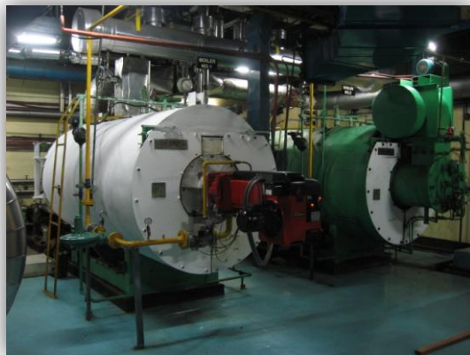
Above: the hotel's two boilers, the first painted and the second in process.
