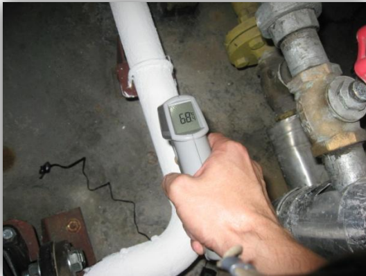
Above: temperature check on painted hot pipe.
