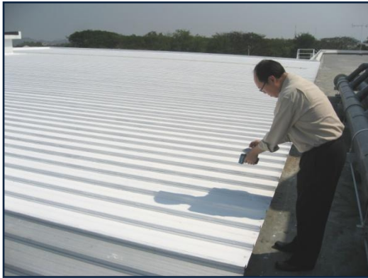
Photo: Carrefour's project manager verifies heat load difference between painted and unpainted roofs.
