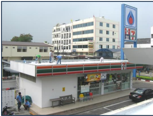
Photo: PTT gas station office's rooftop and 7-11 convenience store's rooftop are now painted and cool.
