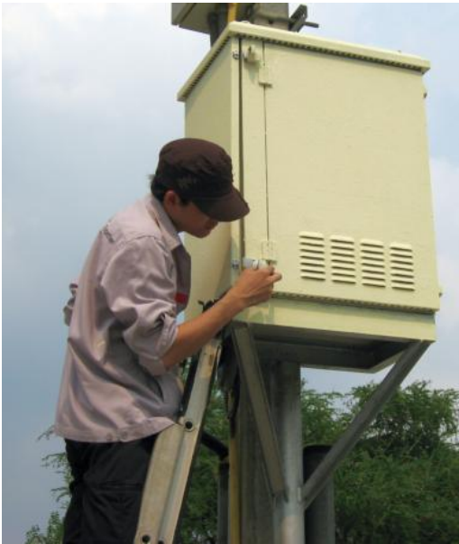
Internet distribution box being painted in light green color: cooler and greener!
