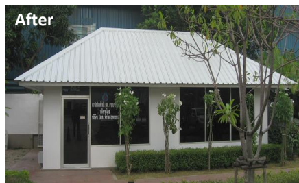
Oct. 2010: now painted with Planet Supra Neo in Light Grey, glossy finish, the office is protected from solar radiations.
