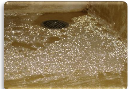
Grout and floors in bathrooms, ...
